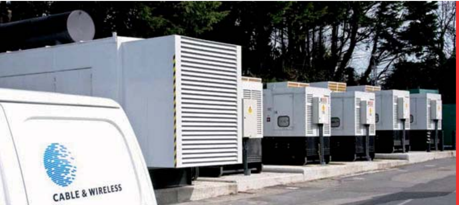
■ PowerBak Generators providing standby power to the Cable & Wireless facility (6x440kVA N+1)
