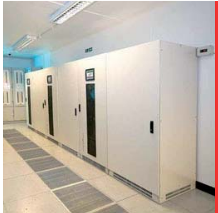
■ Master Plus UPS protection at The Cable & Wireless Data Centre (3x200kVA N+1)
